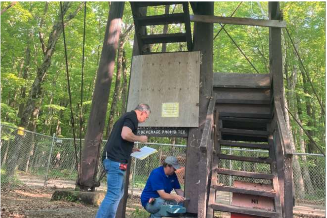
Wood Research and Development's Kim King, senior engineer, left, and James McAdam, level 2 technician, perform an inspection of the Potawatomi Observation Tower on May 30, 2023. Photo by Christie Weber
